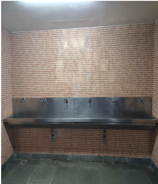
Drinking Water Coolers with RO system, AUMP
